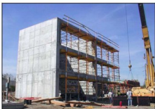
Construction of the specialty manufacturing facility required both damage limiting interior walls and explosion venting exterior walls.
