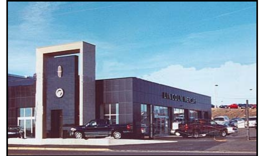
A ceramic tile icon tower marks the Lincoln Mercury showroom. New openings, storefront and aluminum wall panels characterize the renovation.
