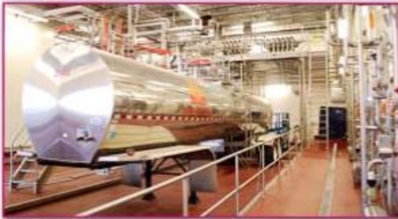
Tanker receiving bay
