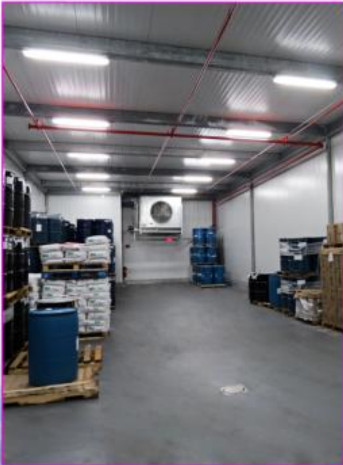
Above: Cold storage warehouse
