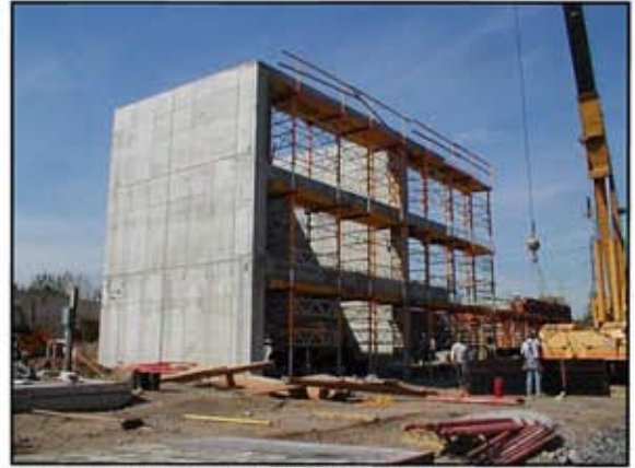
The manufacturing building is an H-3 occupancy constructed with reinforced concrete designed to meet the damage limiting requirements of NFPA 68.
