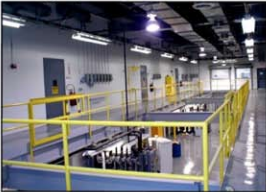
< Interior corridor within the manufacturing building provides access to multi-level production cells, first floor temperature control units, makeup air systems, process utility piping as well as raw material and finish product movement.
