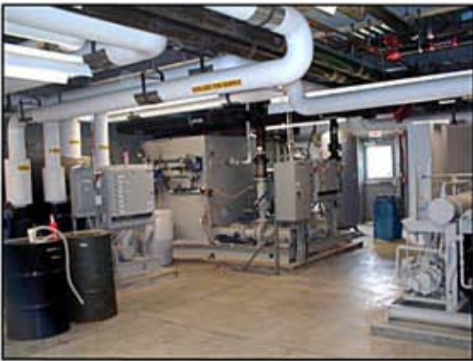
< Mechanical room in manufacturing building which houses the nitrogen generator, nitrogen storage tanks, feed air compressor, dryer for the nitrogen generator, cooling tower and tanks, chiller units and water heaters.
