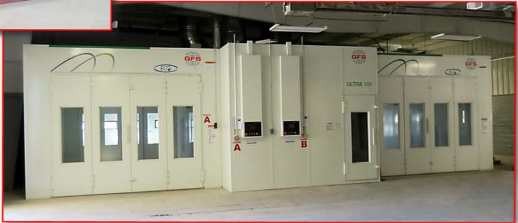
The remodeled paint shop includes two state of the art paint booths separated by the mixing room
